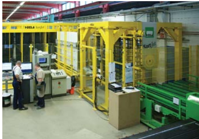
Fig. 03: A swivel conveyor sets the sheet onto the desired edge and transports the sheets from the cutting/ breakout table via loading shuttle into the SortJet slot determined by DynOpt. At the centre, the DynOpt control station - the "brain" of the entire system.
